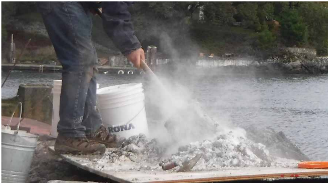
Figure 2. Turning and wetting a dry slaked mortar made using the ‘ring of sand’ method (photo taken by Nigel Copsey; Copsey 2019a: 150; Copsey 2022: 215, Figs. 19–22).
