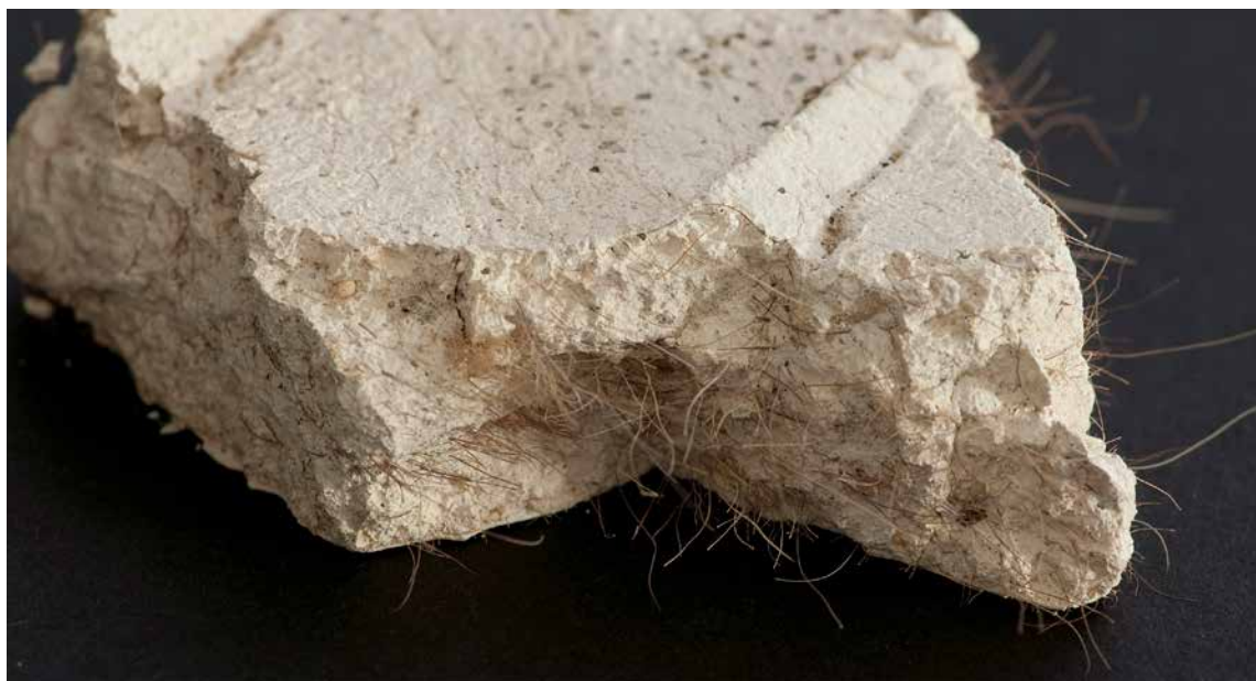
Figure 12. Lime and hair plaster originally applied to riven lath (photo taken by Nigel Copsey).
