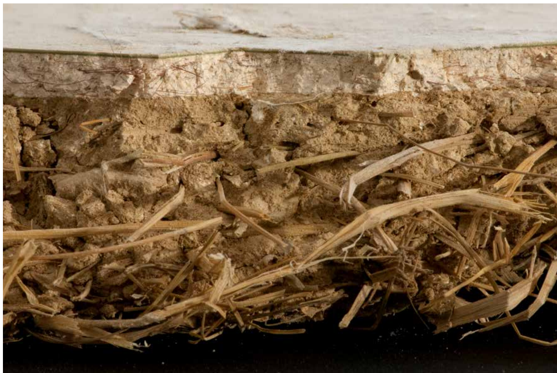
Figure 11. Lime and hair (no sand) mortar over earth-lime backing mortar (photo taken by Nigel Copsey).
