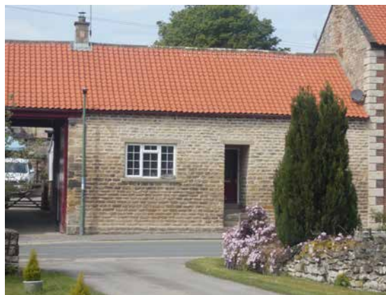
Figure 9. Calcareous sandstone building repointed in November 2023. Fabric saturated by long-term cement pointing. Within 2 days of completion, and regularly through the winter, overnight temperatures fell to minus 10 and minus 15°C. Mortar ratio 1 lime: 1 sand, dry slaked. No frost damage (photo taken by Nigel Copsey).
