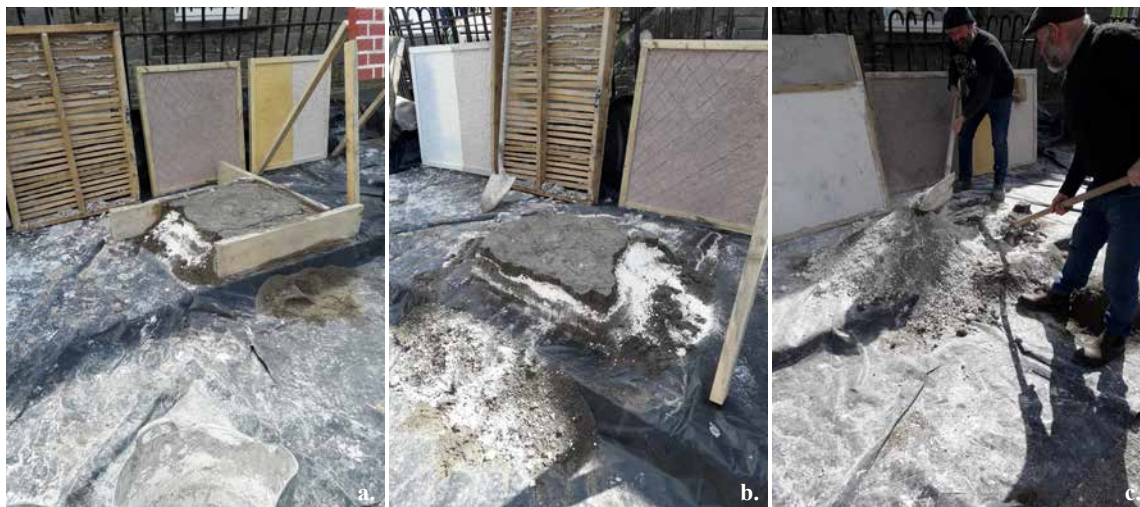
Figure 1. a. A reduced scale dry slake of calcareous sand and lump quicklime after striking of the formwork and b. 24 hours after slaking (normally slaked within a 3.5 metre square formwork, each layer of sand saturated before adding a layer of quicklime, at a proportion of 1 quicklime: 3); c. Damien Condon and Michael Masterton turning the lime and sand together (photos taken by Nigel Copsey).
