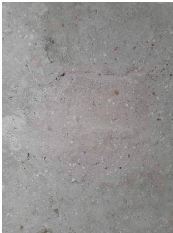
Figure 3. Backing plasters, Schumacher House, c 1870. Haifa, Israel. Maximum size of lime clasts 5mm, indicating sieving of initially dry-slaked lime (photo taken by Nigel Copsey).
