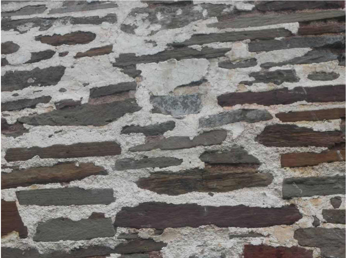
Figure 15. Church of St Clydawg, Clodock, Herefordshire. Very long in situ lime and hair pointing mortars over pit sand bedding mortars, as well as remnant of limewash surface treatment (photo taken by Nigel Copsey).
