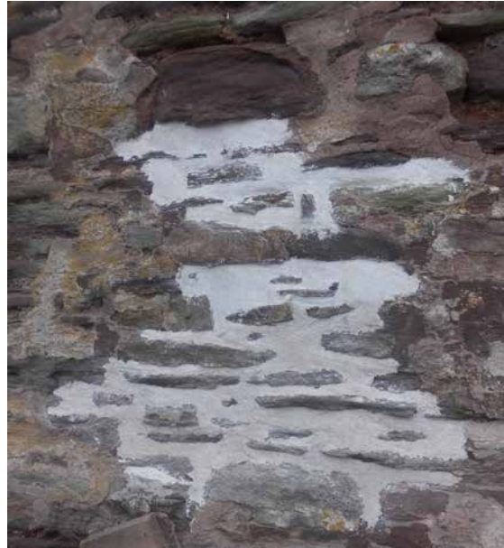
Figure 20. In situ lime and hair pointing trial by the author for English Heritage/Historic England, Longtown Castle Keep, Herefordshire, built with clay-sand mortars c1220 (photo taken by Nigel Copsey).
