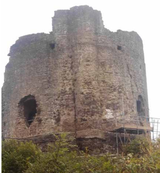
Figure 19. In situ lime and hair pointing trial by the author for English Heritage/Historic England, Longtown Castle Keep, Herefordshire, built with clay-sand mortars c1220 (photo taken by Nigel Copsey).
