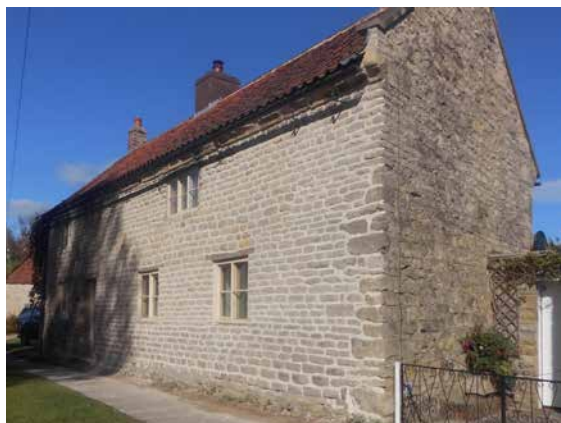
Figure 8. Spring View Farmhouse, Pickering, North Yorkshire. Repointed by the author in October 2024 with a dry slaked, hot mixed pointing mortar, 1.5 non-hydraulic slaked lime: 0.5 fine limestone dust: 0.5 sand and hair. Note the dryness of the repointed facade compared to the gable end wall still, at this time, with its cement pointing (photo taken by Nigel Copsey).
